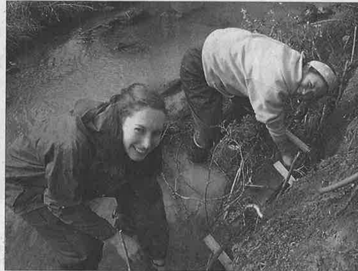
AmeriCorps Water Quality Team members Khann Chov and Meagan Jones plant willow cuttings to prevent bank erosion.
